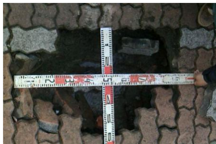
路面陥没 約0.6m×0.9m×0.35m(深さ)
