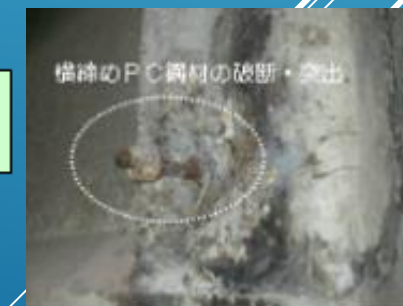
横締め PC 鋼材の突出事例 (Example of protrusion of cross-tensioning PC steel material)
